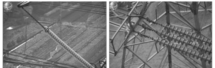
Fig.8 Defects detection for aerial images with green vegetation or angle-steel tower background 图 8 绿色植被和角钢塔背景中绝缘子缺陷检测
