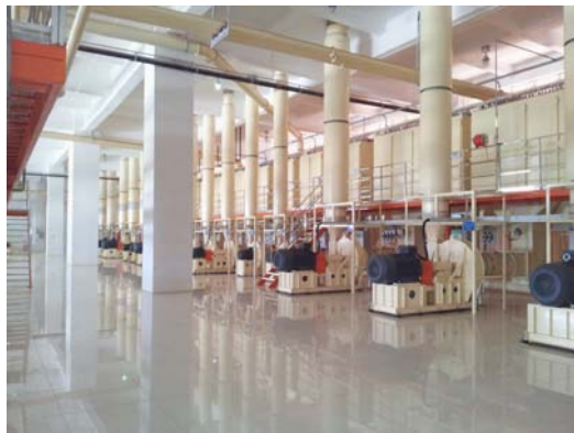
(a) dust removal room
